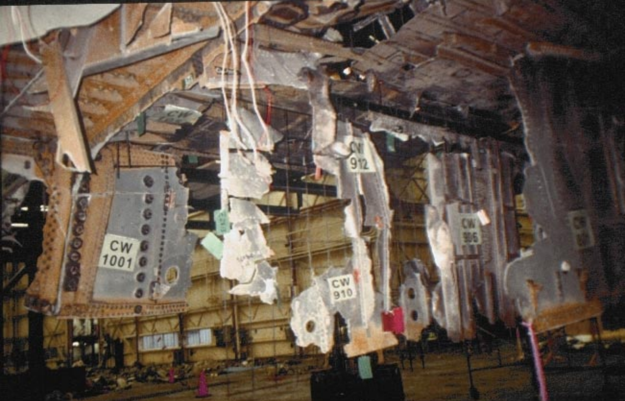
The right hand side of the front of Spanwise beam 1 as viewed from the side, looking at CW 910, 912, and 907. Includes part of the rear spar (1001)
