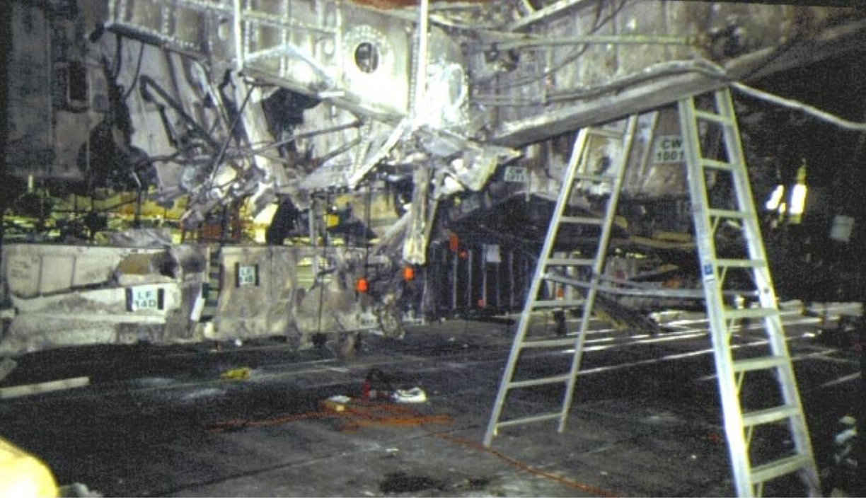
The placement of the keel beam and orange protective caps on the coil rods on March 5
