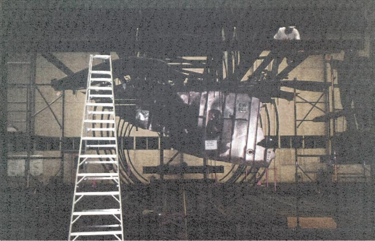
Looking at a portion of the mid spar after assembly on the truss
