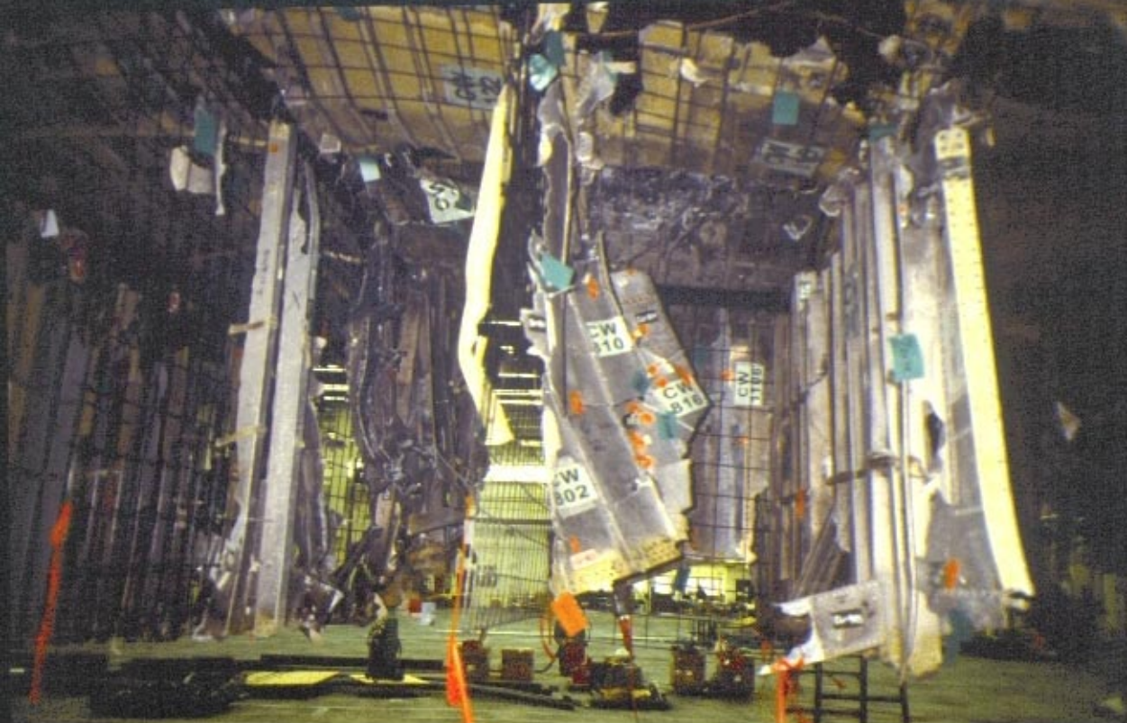
Looking at the mid spar, including CW801, 815, and 816, from the left to the right side
