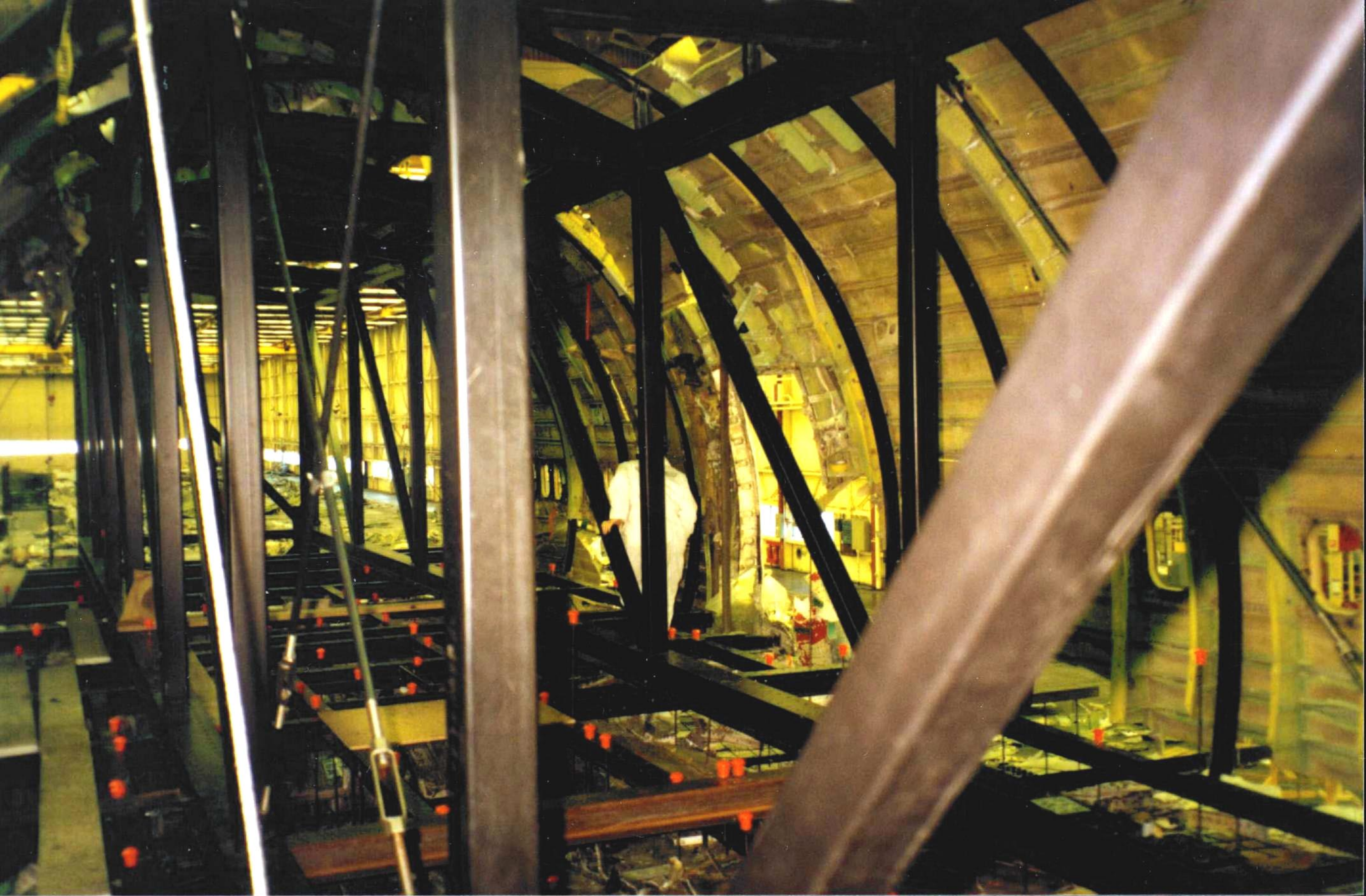
Internal view of the right side looking forward
