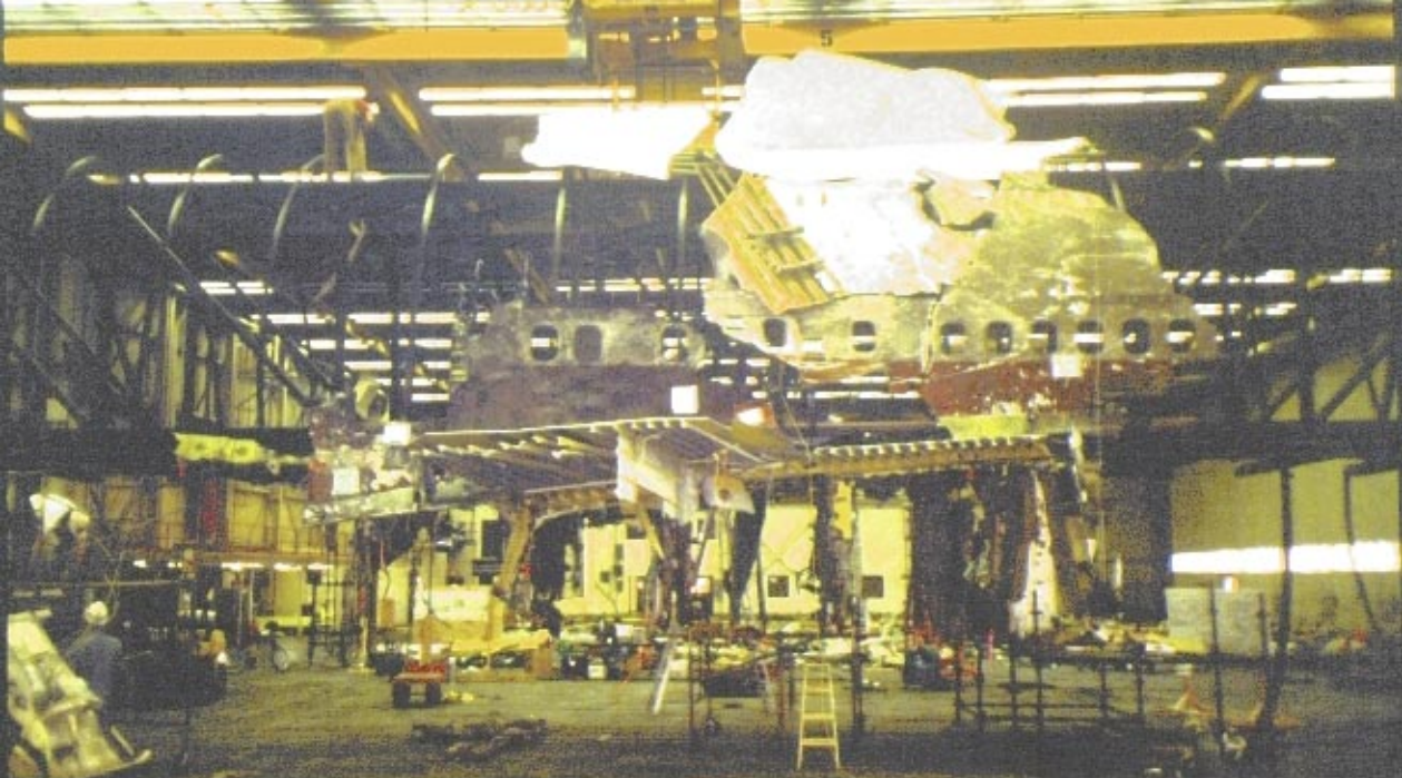
Installation of roof parts as shown from the right side, including RF41 and RF34
