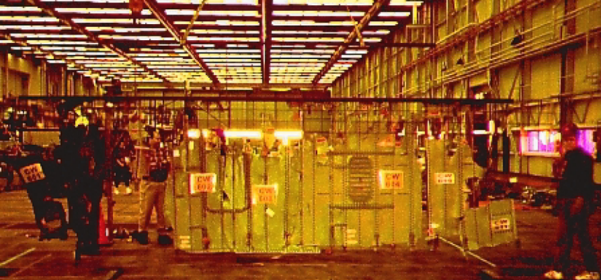
Assembly of span wise beam 3 on mesh, prior to installation on the truss
