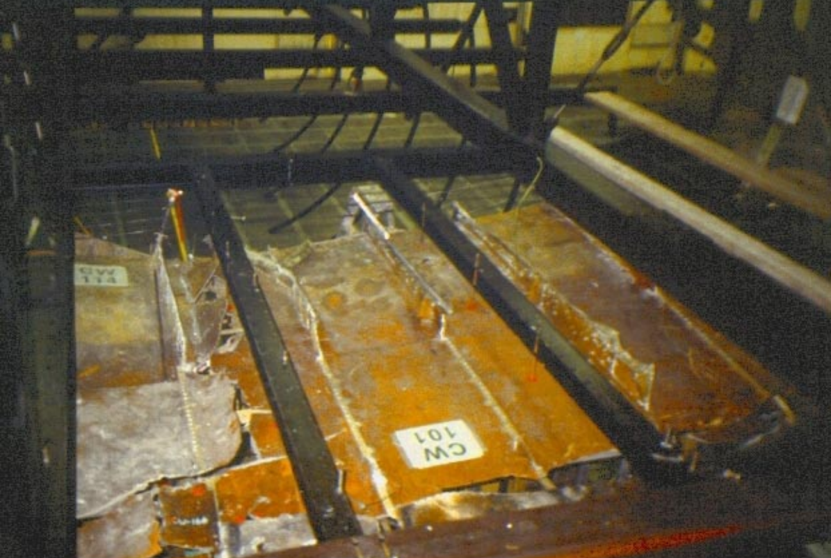
Top of the center wing fuel tank, looking at CW101 and CW114
