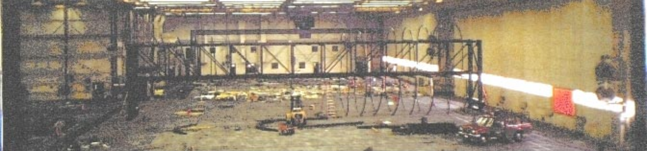
The truss assembled to support the piece of the plane on February 6
