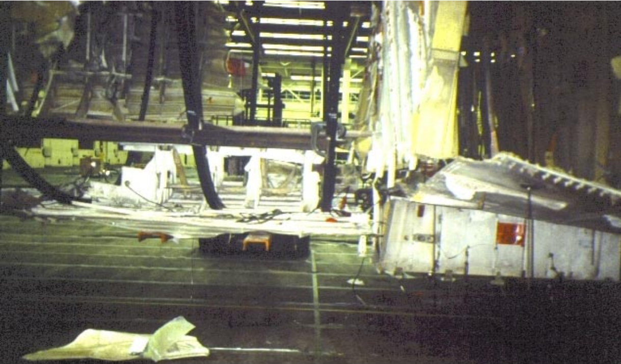
Installation of the bottom of the front cargo bay (LF6A) on March 4 as viewed from the left side
