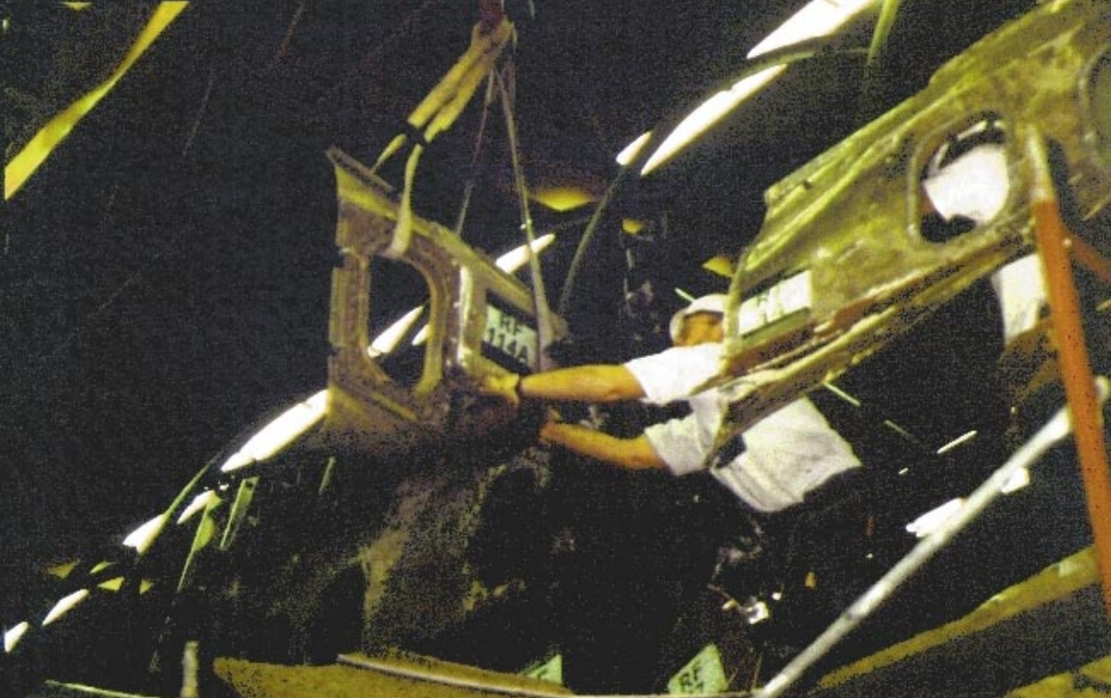
Evaluating RF114A at various locations prior to fastening it to the structure on February 16
